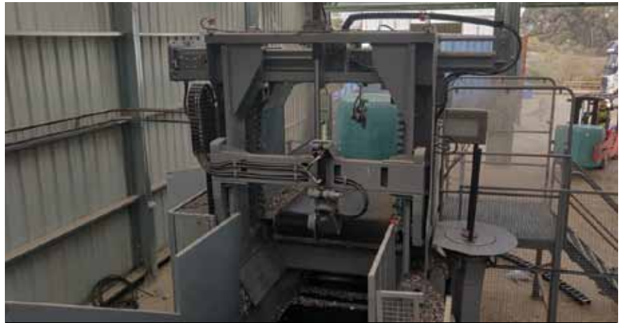
Figure 5: LafargeHolcim Spain invested in an automatic Cross Wrap Bale Opener to improve its waste fuel infeed operation capacity and process automation
